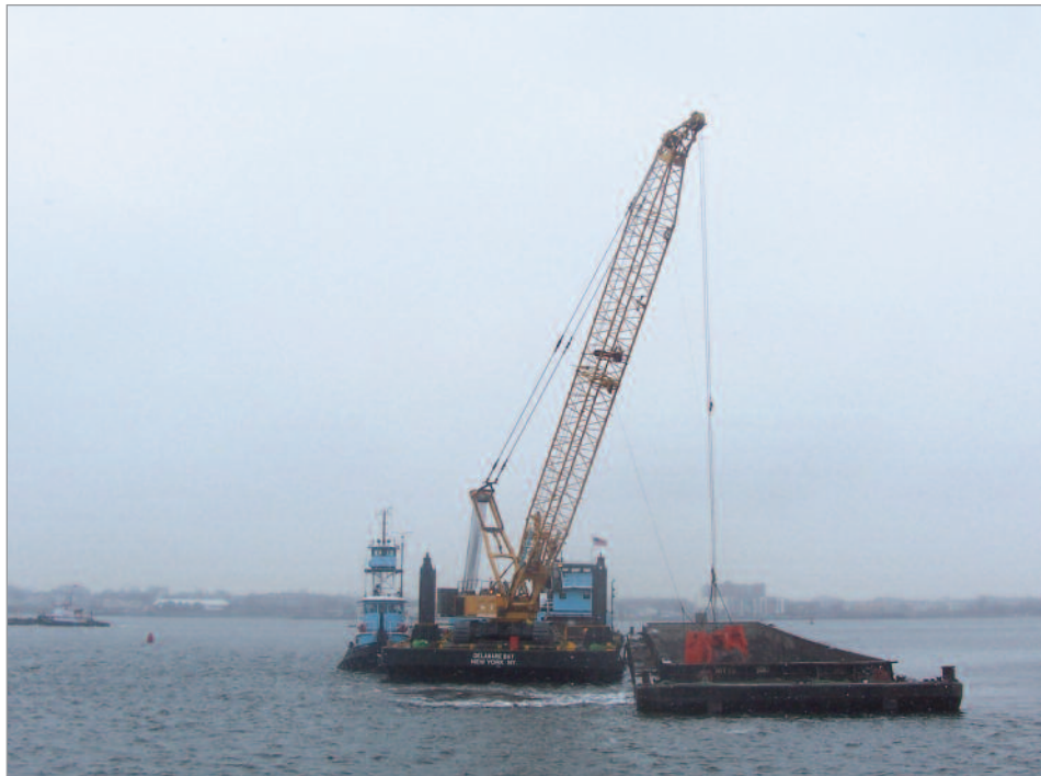
Dredging work continues on the NY & NJ channel improvement project in Elizabeth, NJ.
